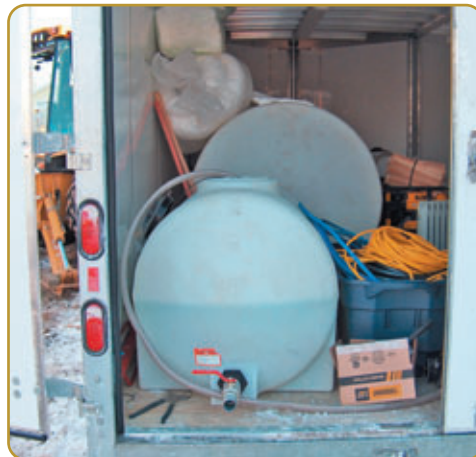
On-site water treatment where the standing water is separated from the oil.
