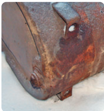
Oil tank clearly showing hole.
