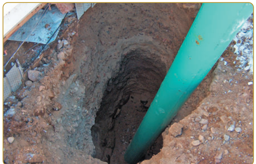
The test pit where the hole was dug directly under the location of the leak from the oil tank.
